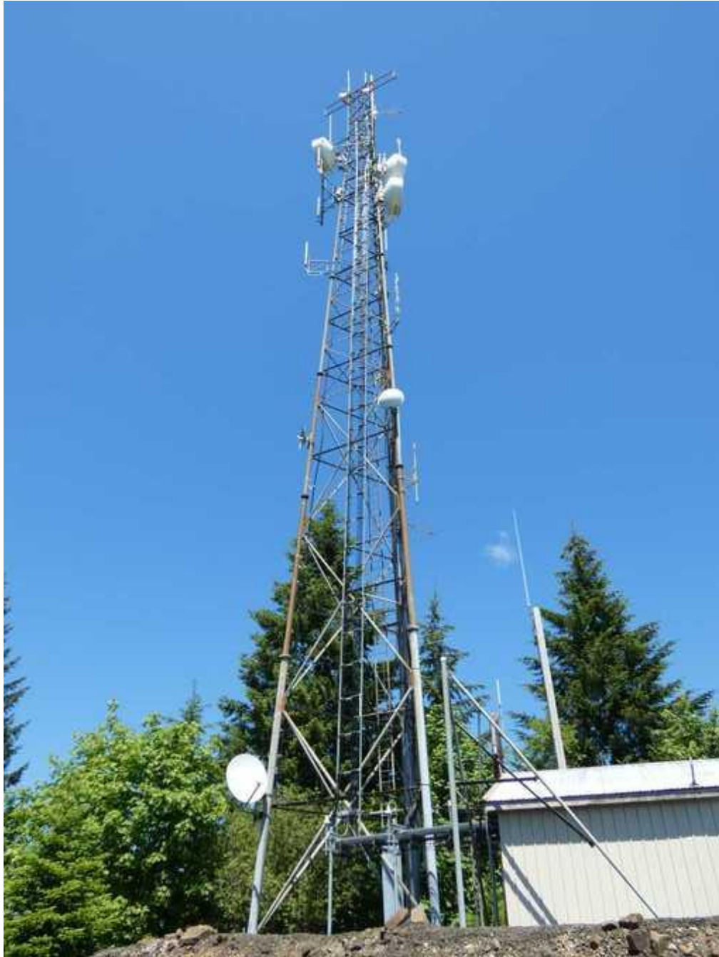
BUSH MTN Tower facing CRAWFORD MT
