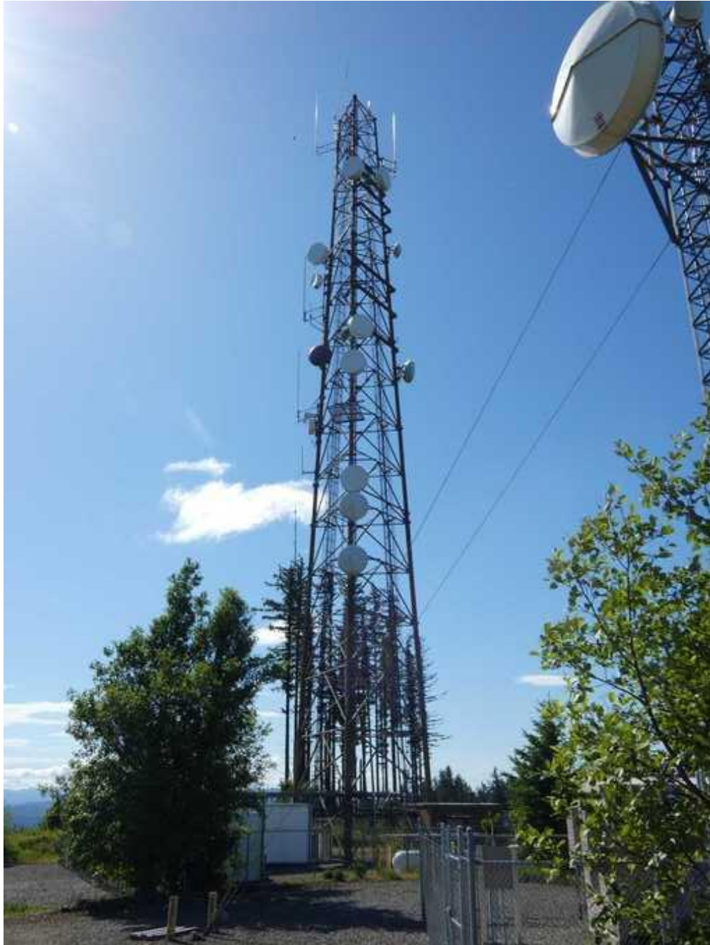
CRAWFORD MT Tower facing SE
